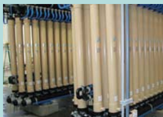
Row River WTP converted from a conventional granular media filtration process to pressurized MF membranes.
